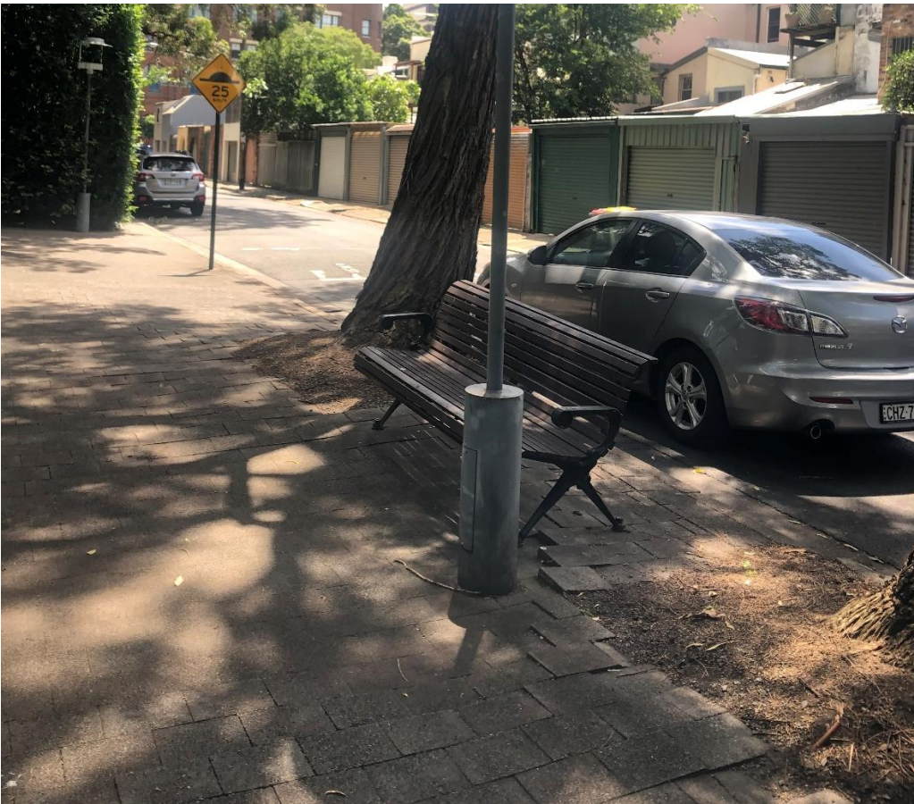
Looking north along McKee Street. Uneven paving along the footpath due to tree roots.
