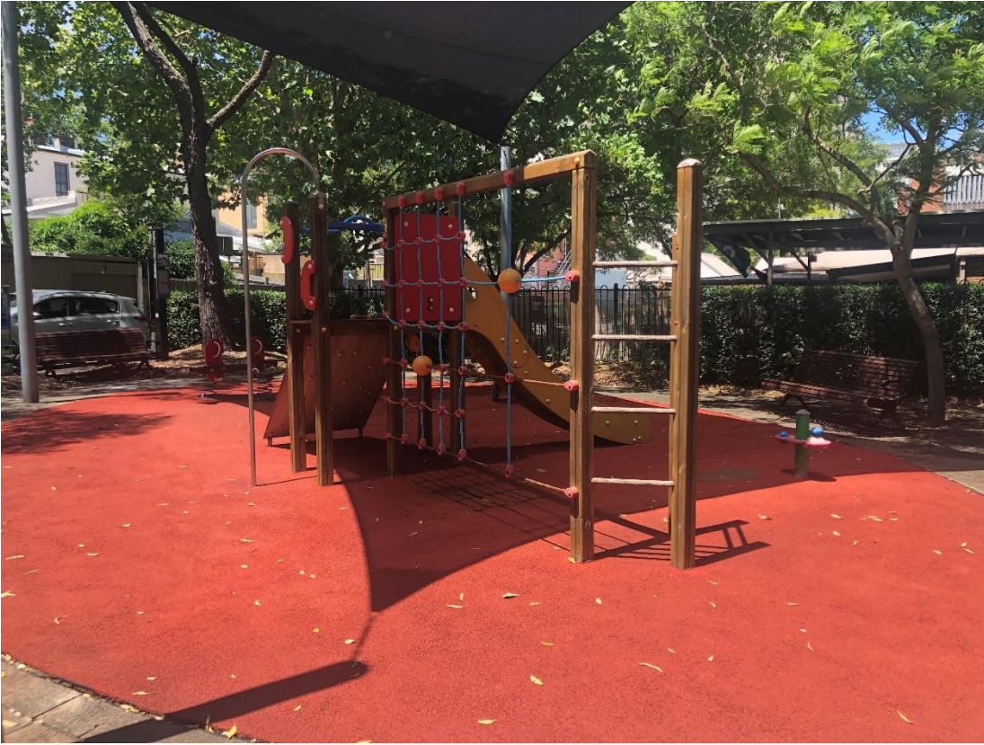
Existing playground in the reserve – play equipment is at the end of its lifecycle; soft-fall is worn and separating from edges. Playground is well shaded from the existing trees and shade structure.
